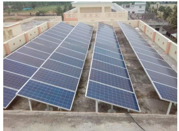
Figure 2: Tilt-mounted solar panels
