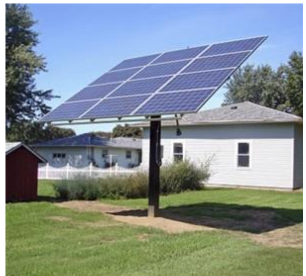
Figure 3: Free standing solar panels
