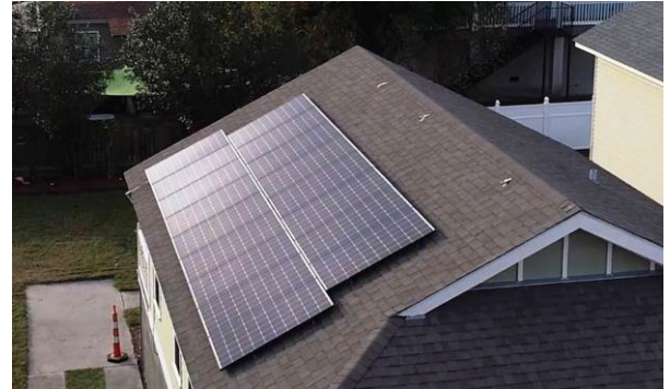
Figure 1: Flush-mounted solar panels
