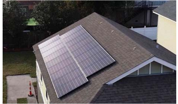
Figure 1: Flush-mounted solar panels
