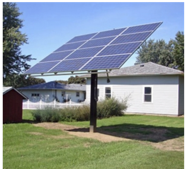
Figure 3: Free standing solar panels
