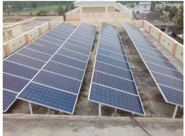
Figure 2: Tilt-mounted solar panels
